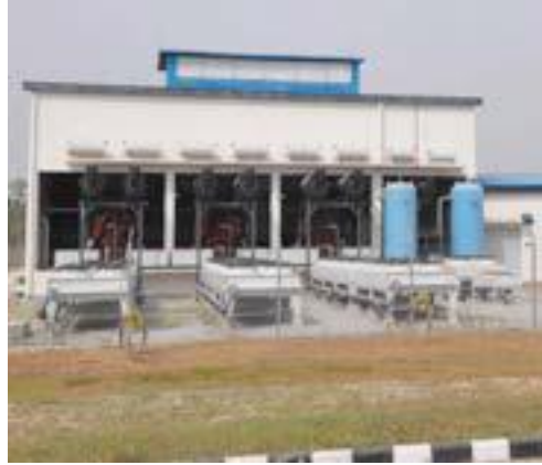
Lekki Free Trade Zone 12MW Generation Project
